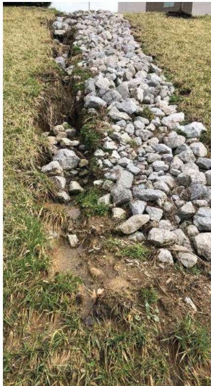
Stormwater erosion has formed a gully on the left side of the forebay.
