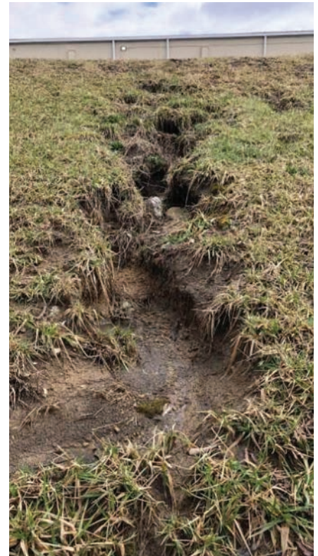
Concentrated stormwater flow has eroded sediment from the embankment, forming a gully.
