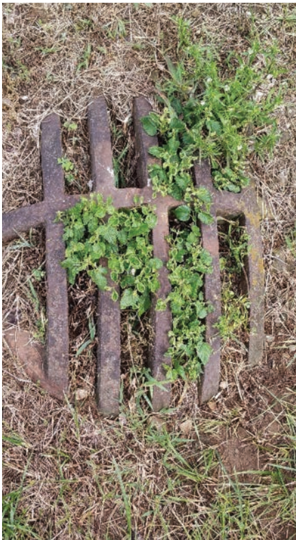
The outlet is being buried in sediment and vegetation.
